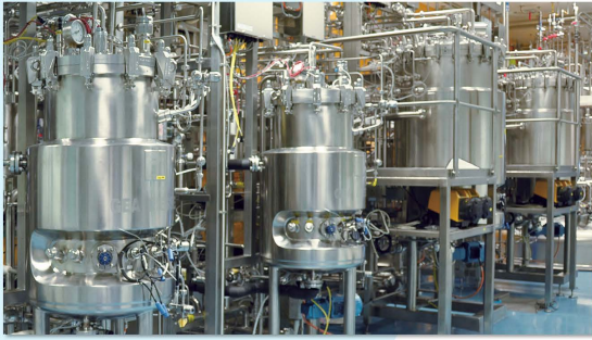
Fermenter/Digestor Production Facility
